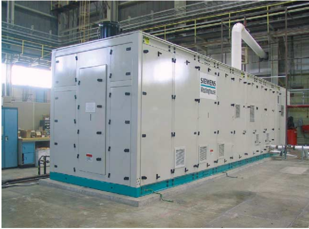
Fig. 5. Siemens Westinghouse's 250 kW size atmospheric pressure CHP system.
