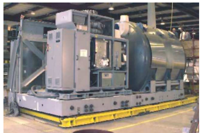
Fig. 8. Siemens Westinghouse 330 kW pressurized SOFC/turbine hybrid system for RWE, Germany.
