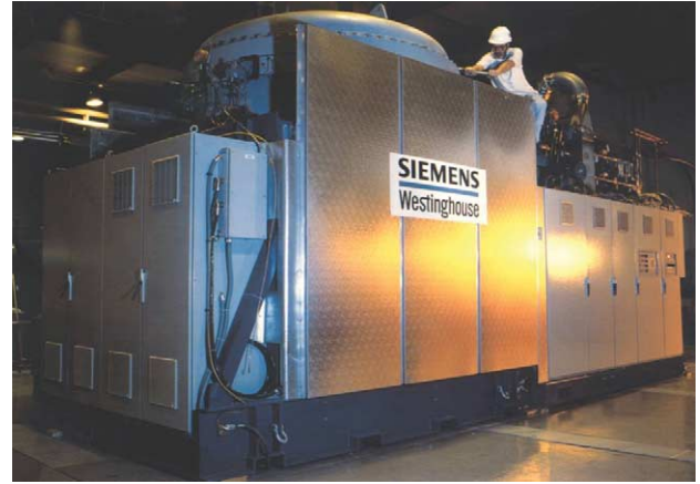
Fig. 7. Siemens Westinghouse's 200 kW pressurized SOFC/gas turbine hybrid system.
