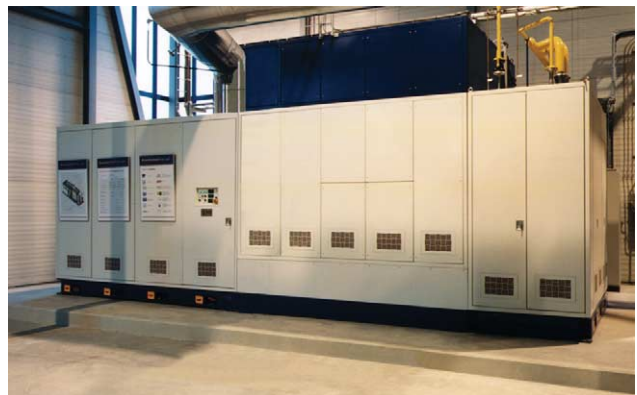
Fig. 4. Siemens Westinghouse’s 100 kW size atmospheric pressure CHP system.
